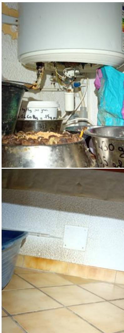
Photo Alimentation Electrique
