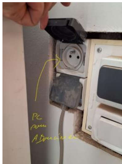
Photo Alimentation Electrique
