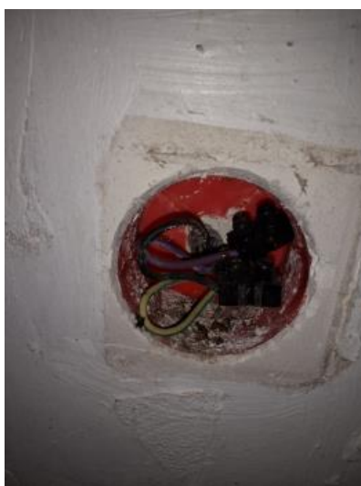
Photo Alimentation Electrique
